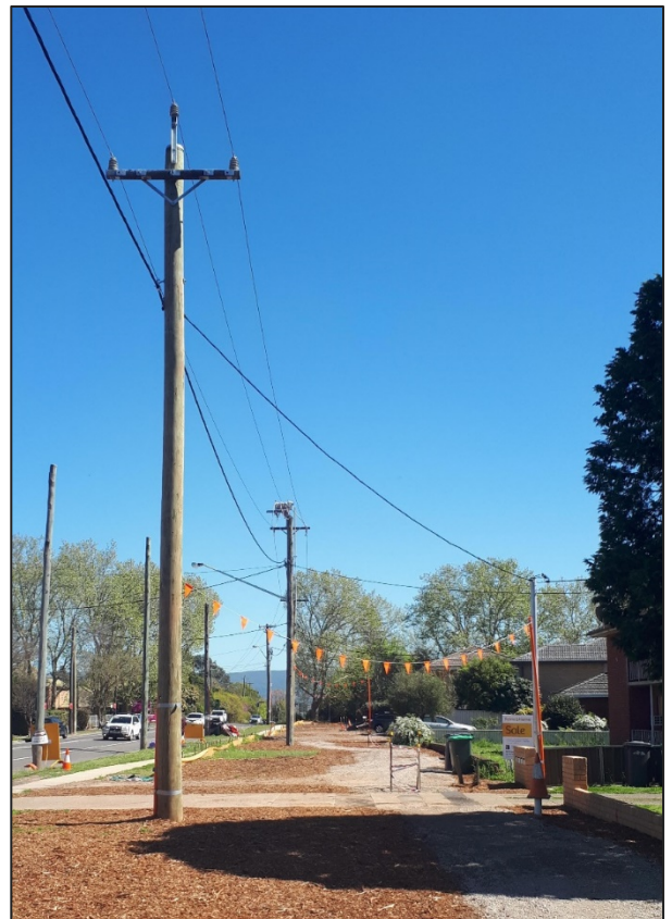
Image: view of March Street after relocating utilities for the wider intersection at March and Bosworth streets.
