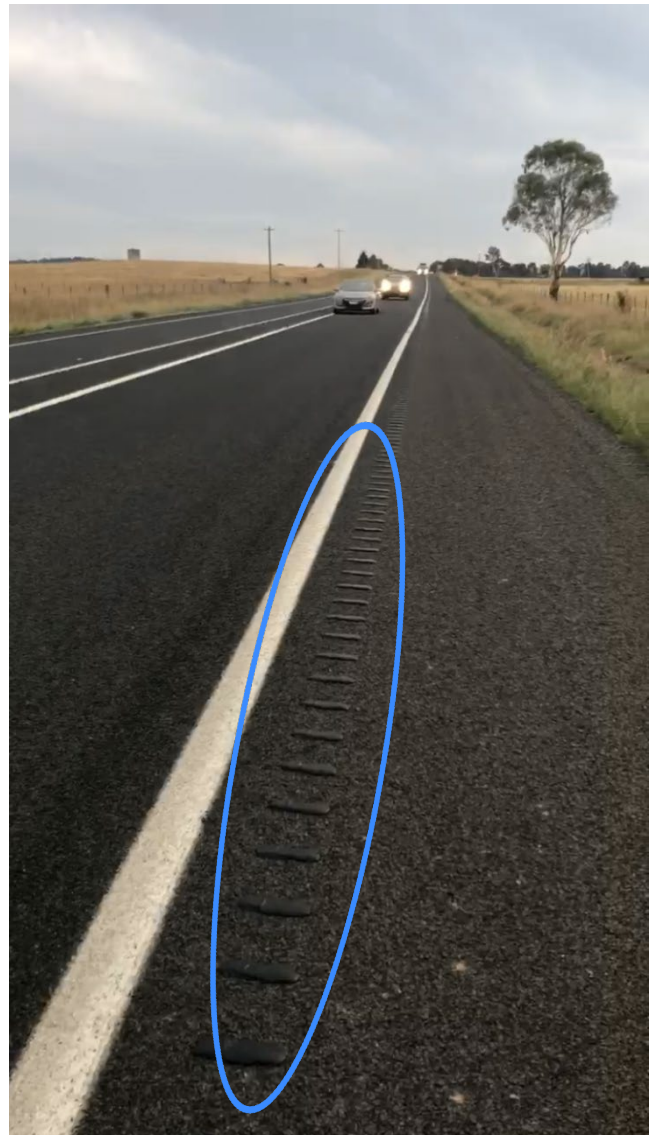
Black ATLM installed on the New England Highway.
