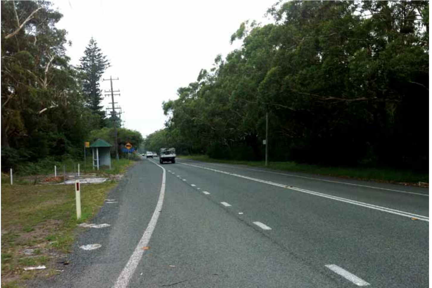
Nelson Bay Road is being duplicated with safe access for adjoining properties and bus bays
