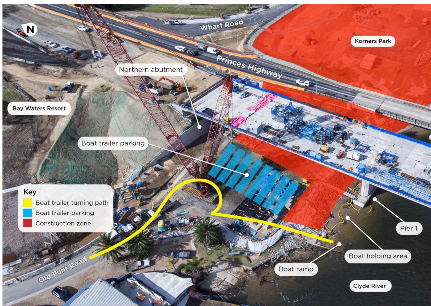
Old Punt Road boat ramp including boat trailer parking locations, boat trailer turn-around path, and pedestrian access.
