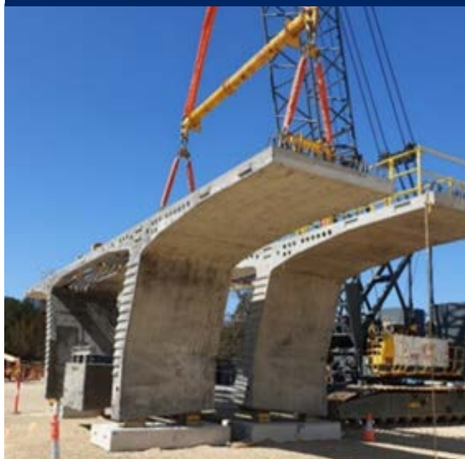
Concrete bridge segments produced at the project's pre-cast facility south of Mogo.
