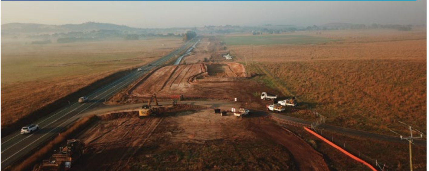
An aerial image of the first stage of the Barton Highway duplication project
