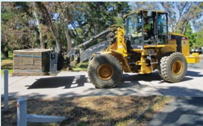
Salvage removal of the old tanning pit from the 'Dellwood' property during January 2021
