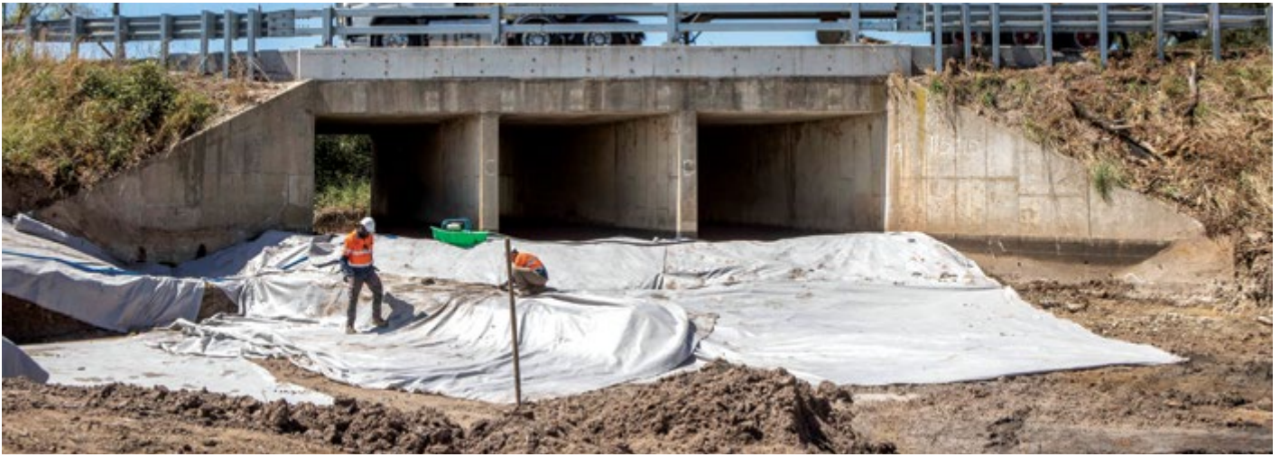
Preparation work under way for the installation of precast drainage structures at Little Bedulluck Creek
