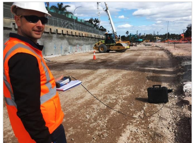
Image: vibration monitoring in western carriageway
